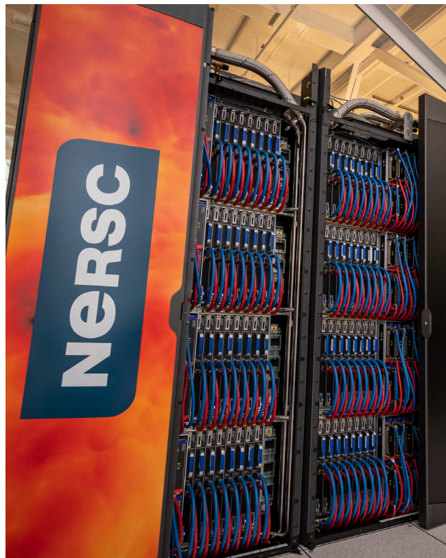
Figure 3. An inside view of Perlmutter reveals that the compute cabinets are liquid-cooled. Redundancy in cooling units is provided as needed. All non-compute nodes housed in service cabinets are air-cooled.
